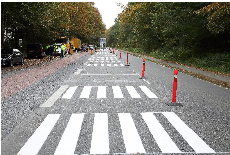
Figure 1. The test field in Denmark at the time of application.
